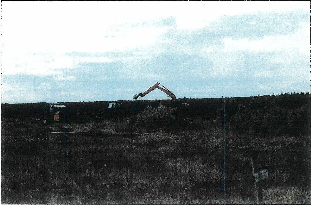
Figure 5: EVIDENCE OF POTENTIAL UNAUTHORISED ACTIVITY 07/06/21
